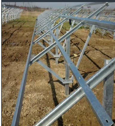
Typical Ground Mounting
