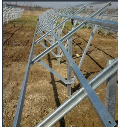
Typical Ground Mounting
